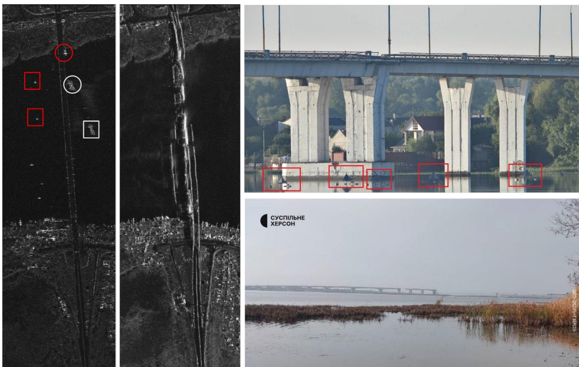
Picture n. 4: The two images on the left are high-resolution SAR imagery acquired on different days. In the first image, various targets can be identified over the river. In the second image, damage to certain parts of the bridge is visible. On the right side there are images retrieved from online newspapers, depicting the presence of floating radar reflectors and the partial collapse of the bridge. This OSINT information were essential for classifying the targets and features visible in the SAR images.
